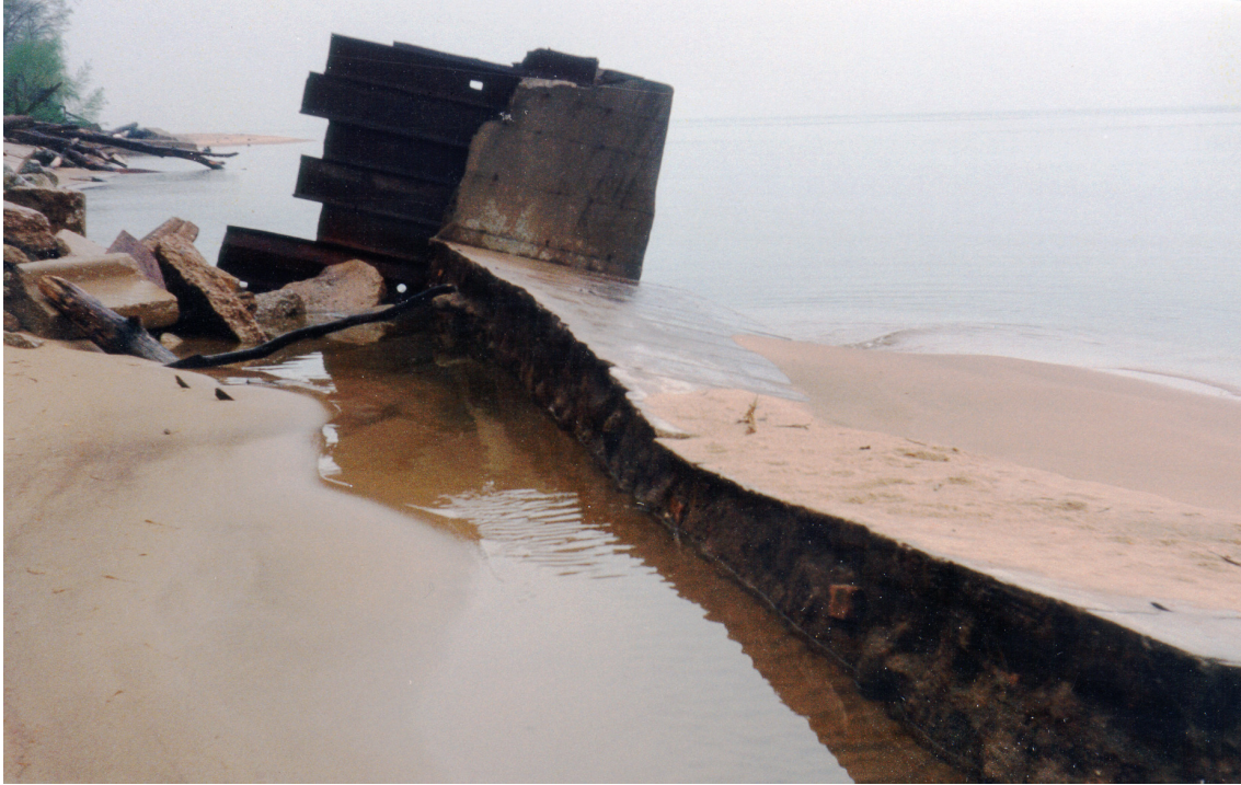
Figure III-5-27. A toppled concrete seawall along the Lake Michigan coast of Berrien County. Failure probably resulted from undermining of the underlying glacial till foundation, April 1991
